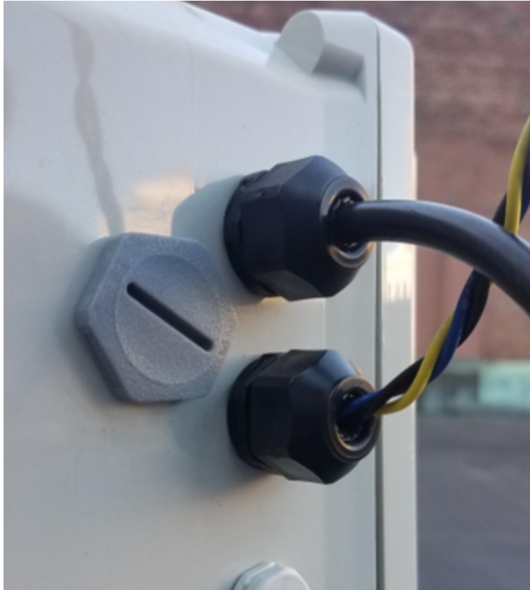
Fig 9: Cord grips tightened down
