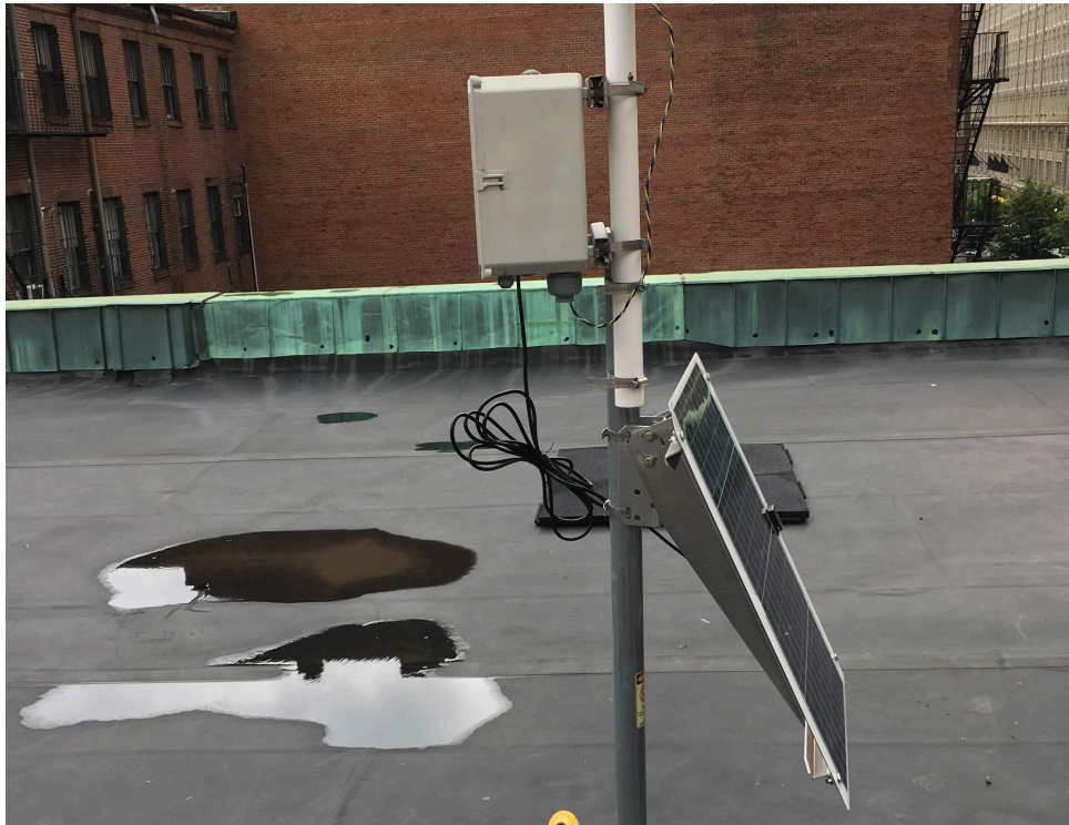
Fig 5: Opti Monitoring Panel and solar panel attached to a pole
