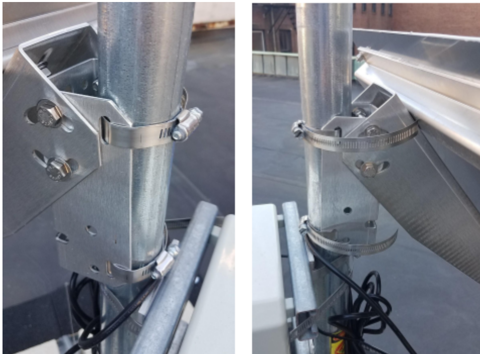
Fig 6: Solar panel mount close-up
