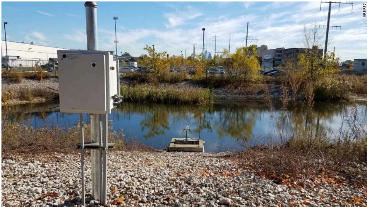
Figure 1: Opti active control installation
