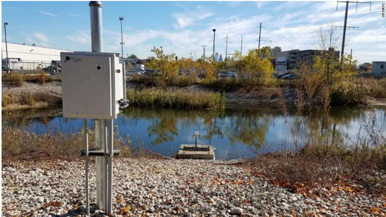
Figure 1: Opti active control installation
